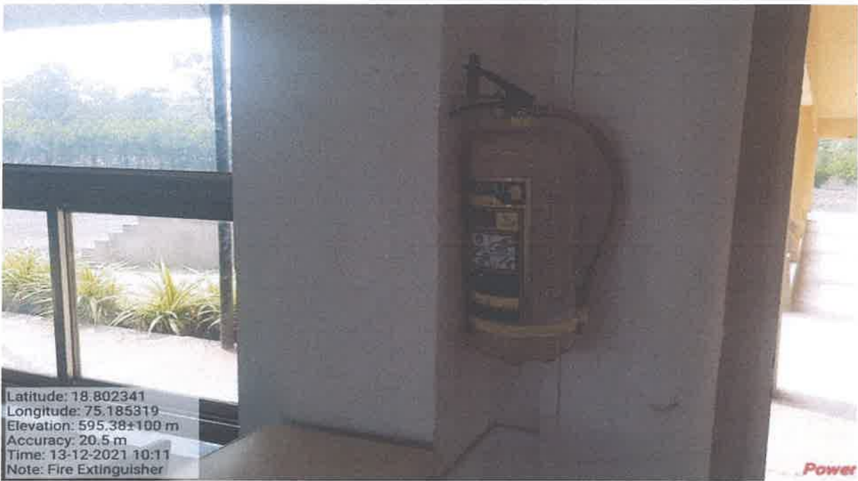
Fire Extinguisher System of Library
