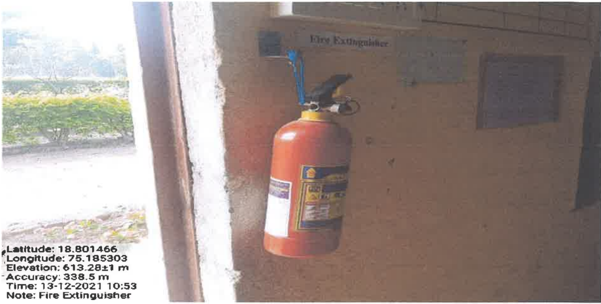
Fire Extinguisher System of Department
