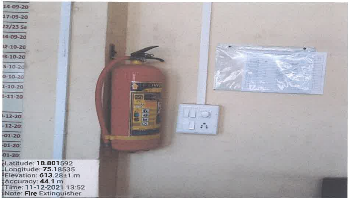
Fire Extinguisher System of Office
